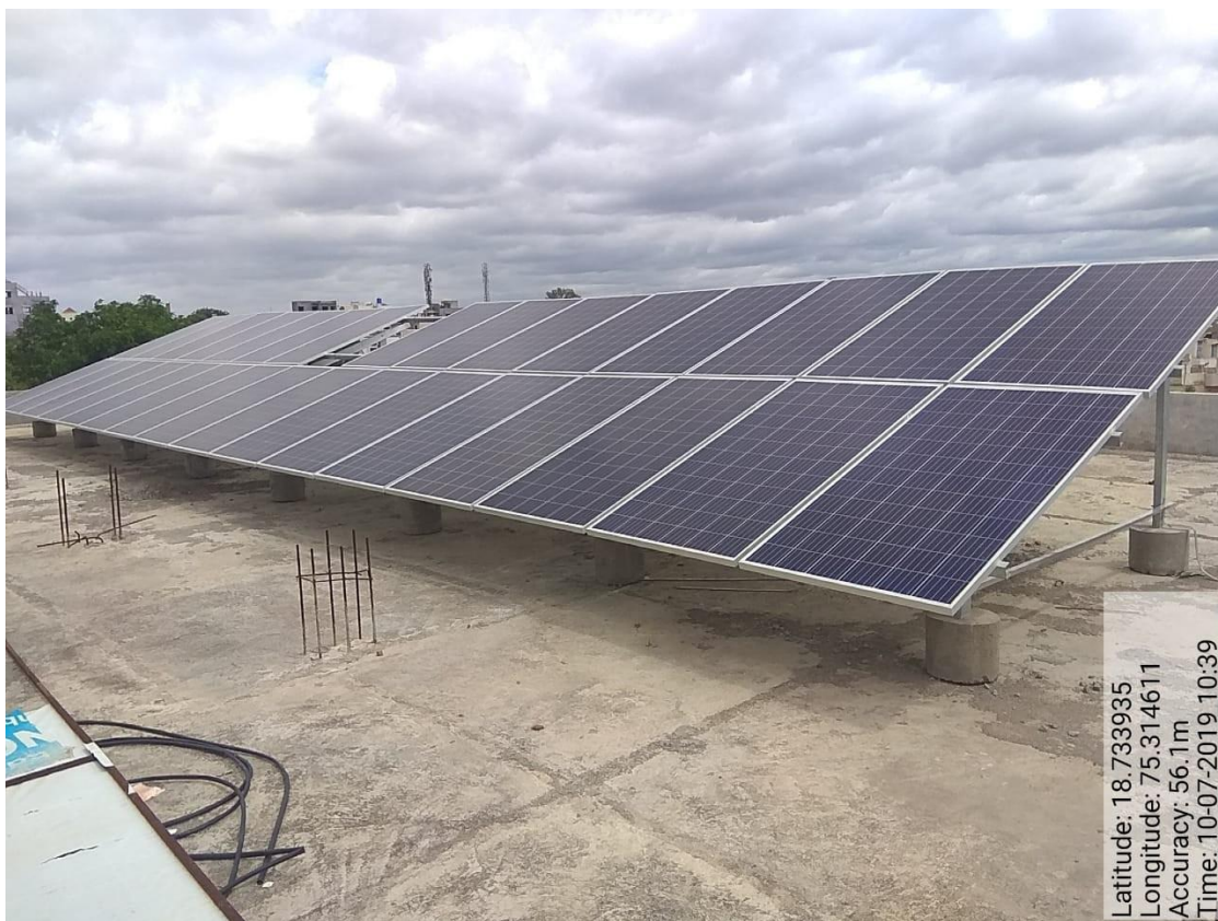
Photo: 10 kW solar roof top on institute building roof.
